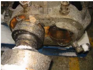
Bearing Caps Both are damaged /worn
