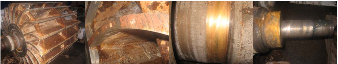
Rotor Scoring to rotor face Worn packing sleeve Worn bearing diameters Body 1 (smaller section)
