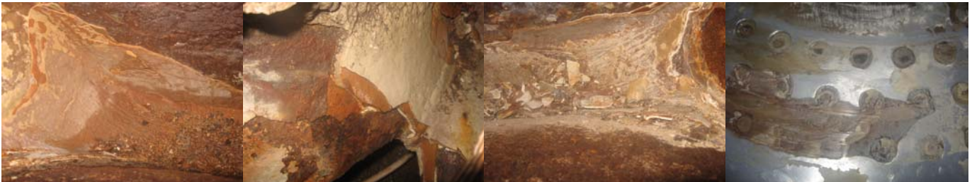
Scale build up in header internals, Rotor and anti cavitation holes
