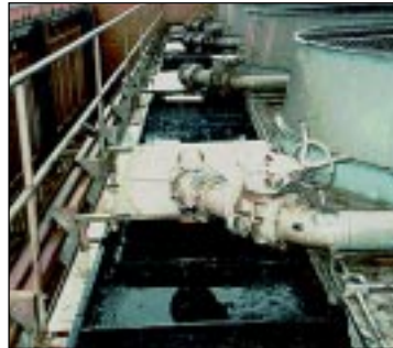
COOLING TOWER PANS
